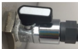
DRAIN VALVE OPEN
